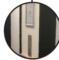
Existing lift control panels to remain and be placed onto wall panels where possible (panels to be 25mm thick).
